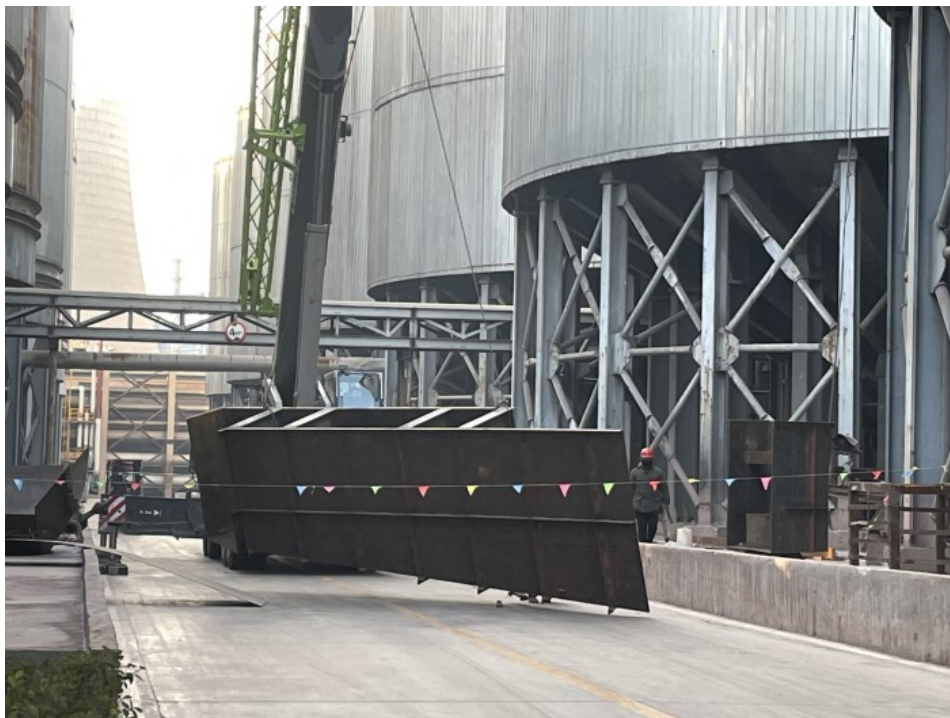
Figure 7. New high-efficiency settler installation on site.
